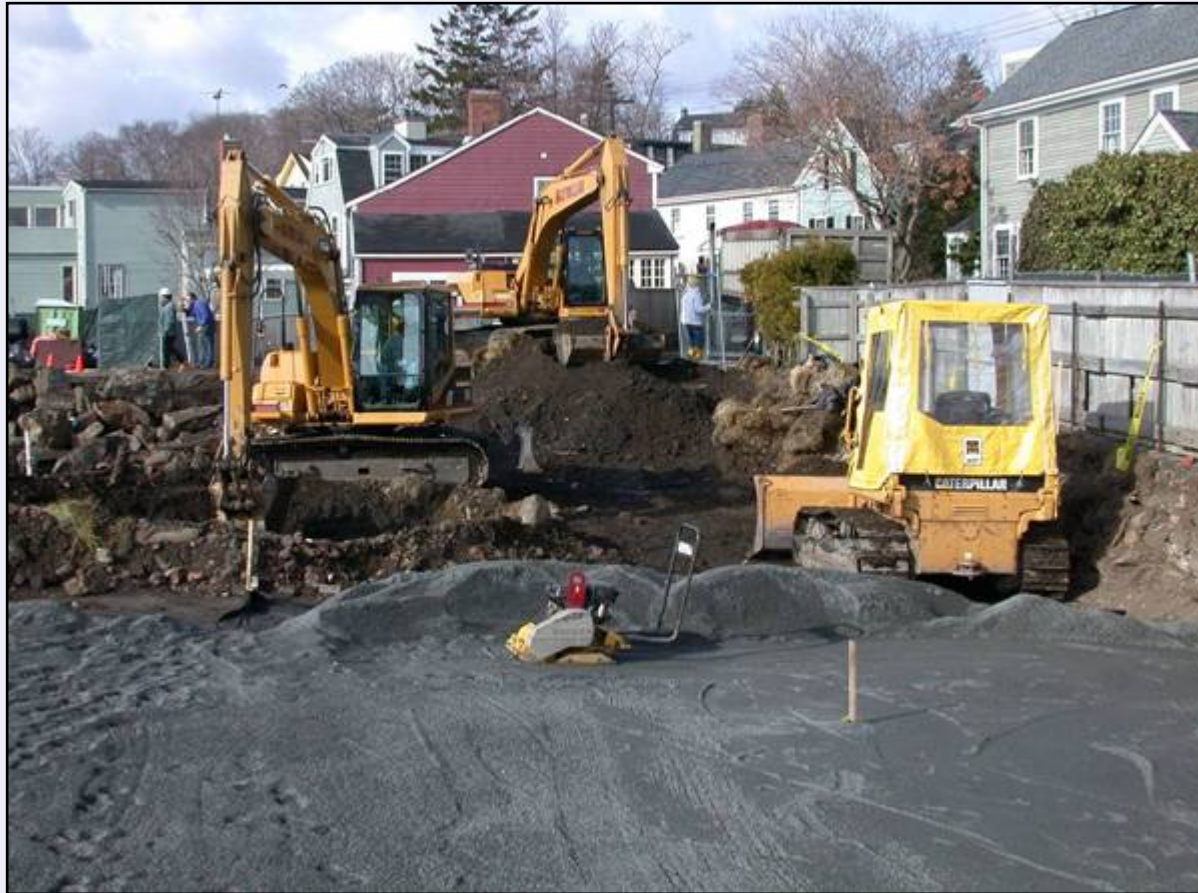
Photo Courtesy of National Grid
